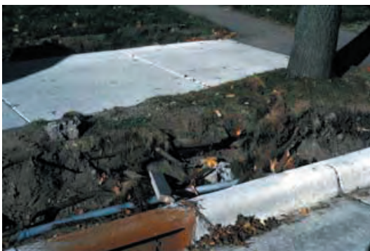
Figure 5.27. This tree has experienced damage to two sides of the root system and surface root loss due to re-construction activities. An older sidewalk restricts the roots on a third side of the root system, making this tree a prime candidate for failure.
