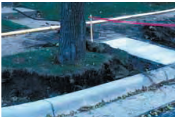
Figure 4.2. Tree with excessive root severing caused by curb and sidewalk reconstruction damage. Root severing can compromise the structure of a sound, healthy tree and increase its susceptibility to windthrow during wind loading events.
