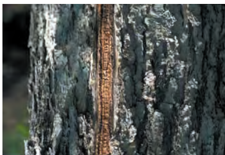
Figure 3.65. Seams are fully compartmentalized. If internal decay is present, check shell thickness.
